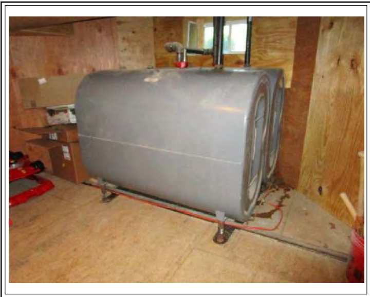
Basement - Oil Tanks
