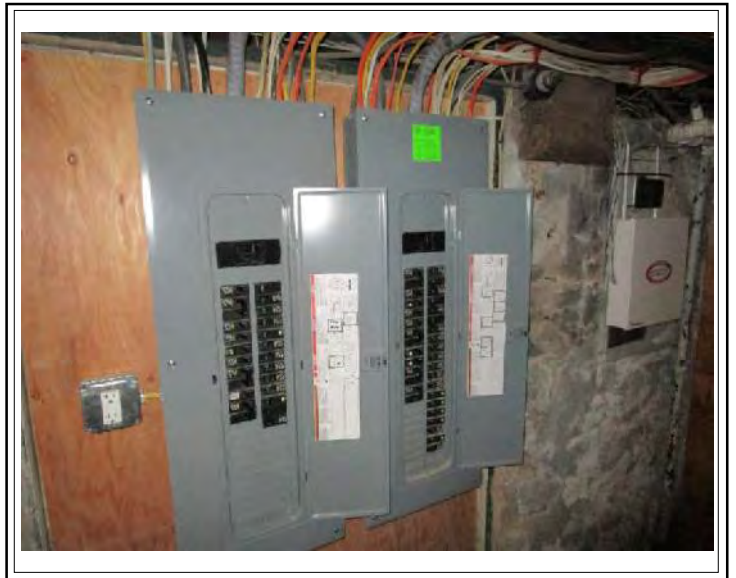
Basement - Electric Panels
