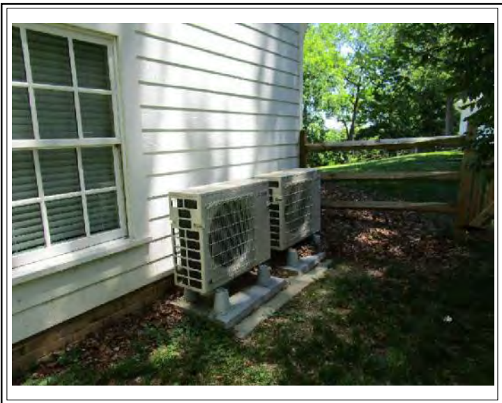
5/Car Detached Garage - Condensers
